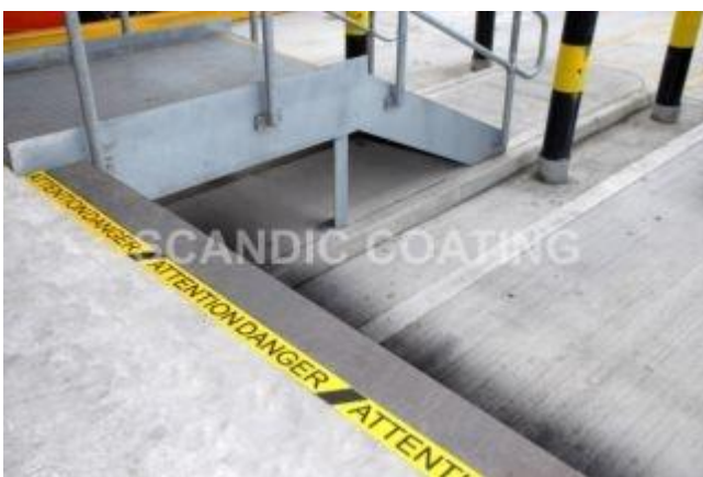
H3416 ATTENTION DANGER being applied E JPG file, 862 KB
